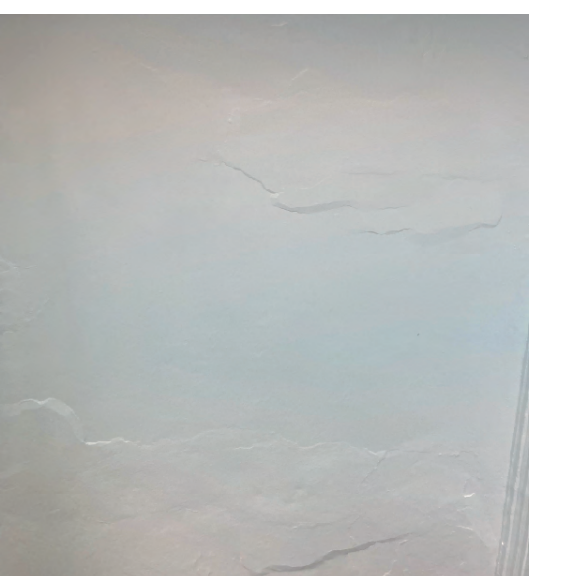
13) Spalling Concrete Cover of Ceiling
