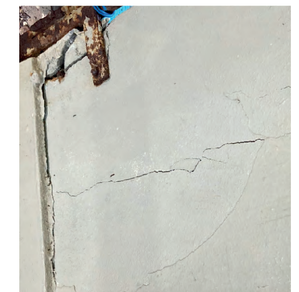
1) Spalling Concrete Cover of Wall
