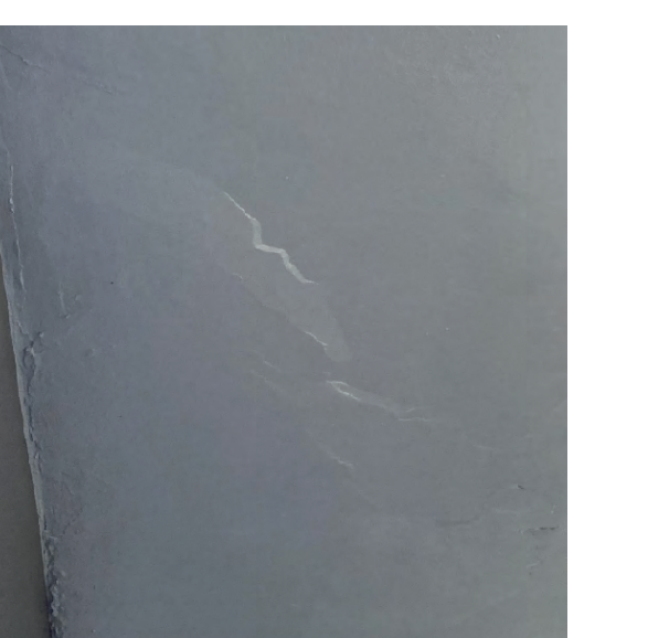
18) Spalling Concrete Cover of Ceiling
