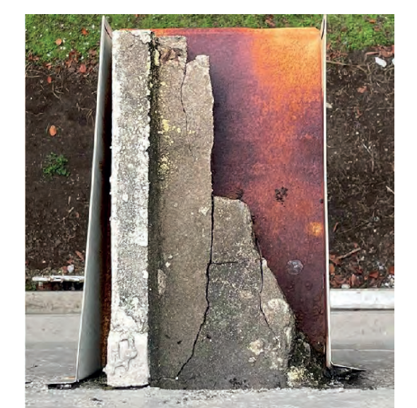
20) Rusted & Broken Storm Water System
