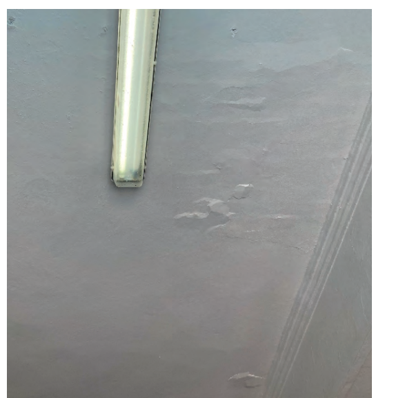
12) Spalling Concrete Cover of Ceiling
