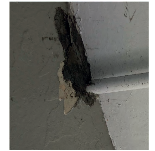
6) Spalling & Delaminated Concrete Cover of Wall
