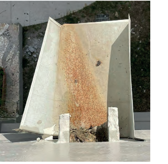
8) Loose Hanging Storm Water System
