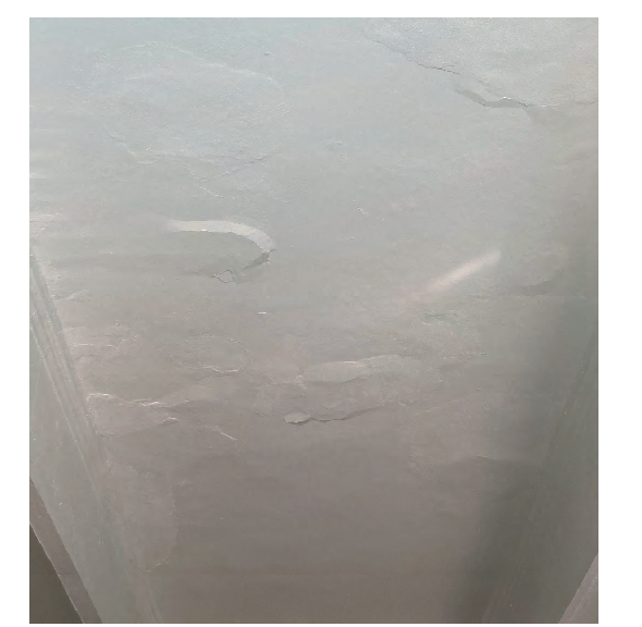
11) Spalling Concrete Cover of Ceiling
