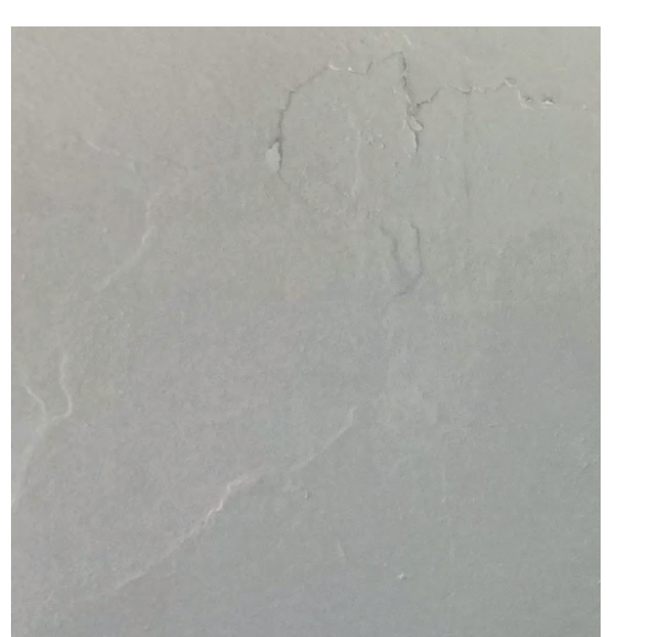
19) Spalling Concrete Cover of Ceiling
