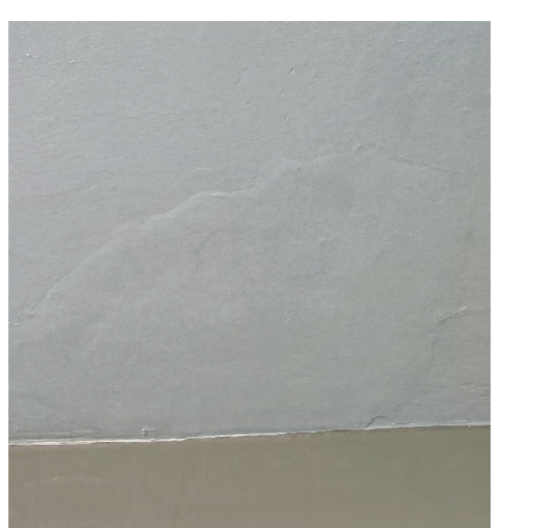
17) Spalling Concrete Cover of Ceiling
