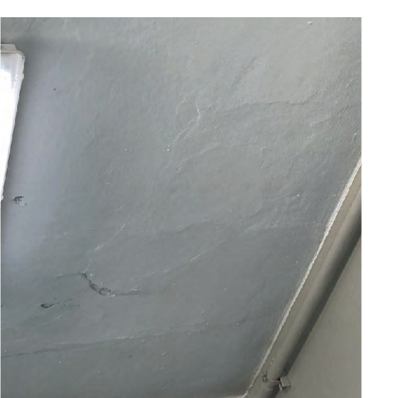
23) Spalling Concrete Cover of Ceiling
