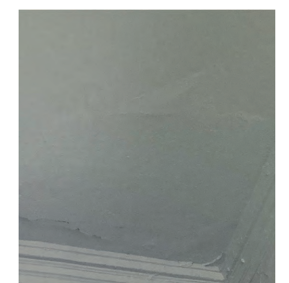
15) Spalling Concrete Cover of Ceiling
