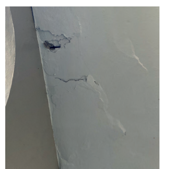
21) Spalling Concrete Cover of Ceiling
