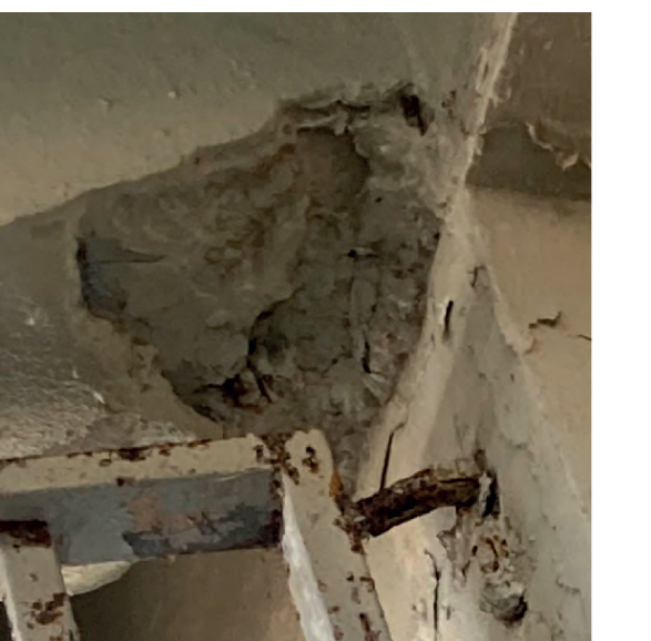
3) Spalling & Delaminated Concrete Cover of Ceiling
