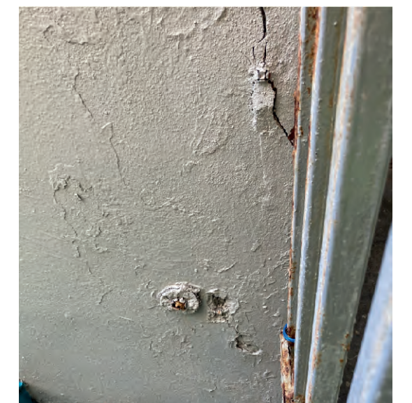
2) Spalling Concrete Cover of Wall
