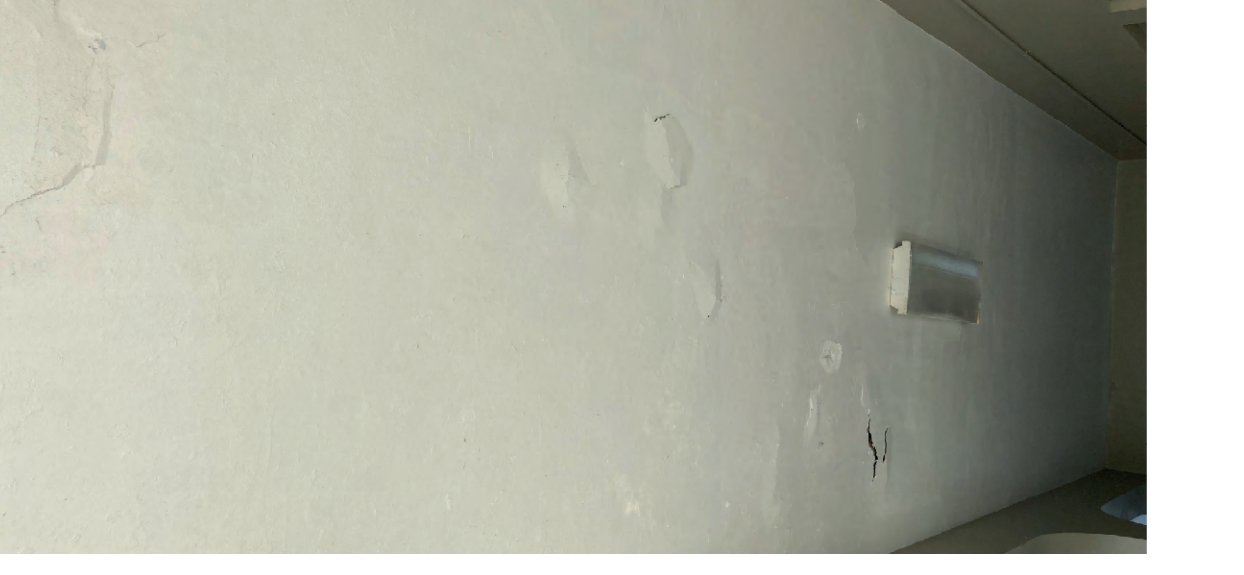
9) Spalling Concrete Cover of Ceiling
