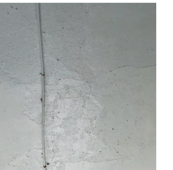
5) Spalling Concrete Cover of Ceiling
