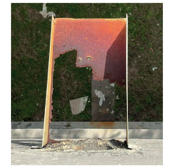
10) Broken Storm Water System
