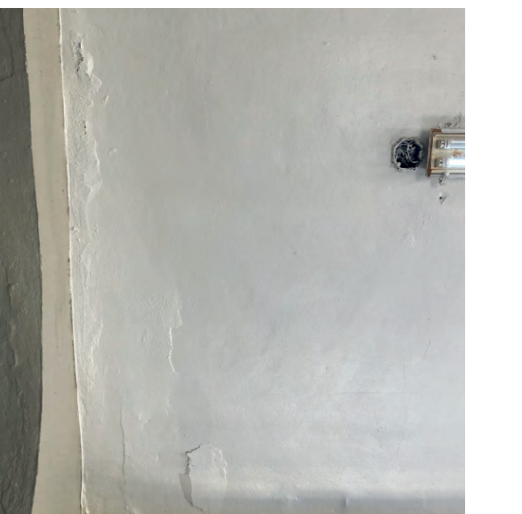
4) Spalling Concrete Cover of Ceiling
