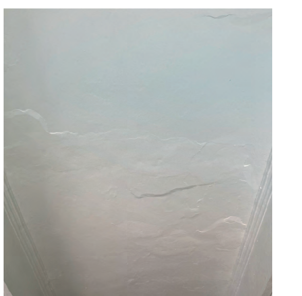
14) Spalling Concrete Cover of Ceiling
