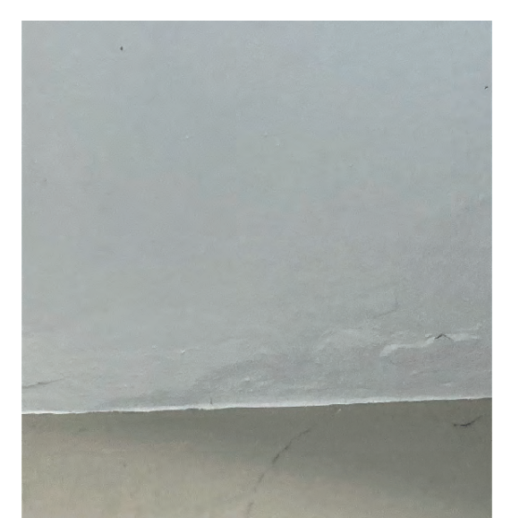
16) Spalling Concrete Cover of Ceiling
